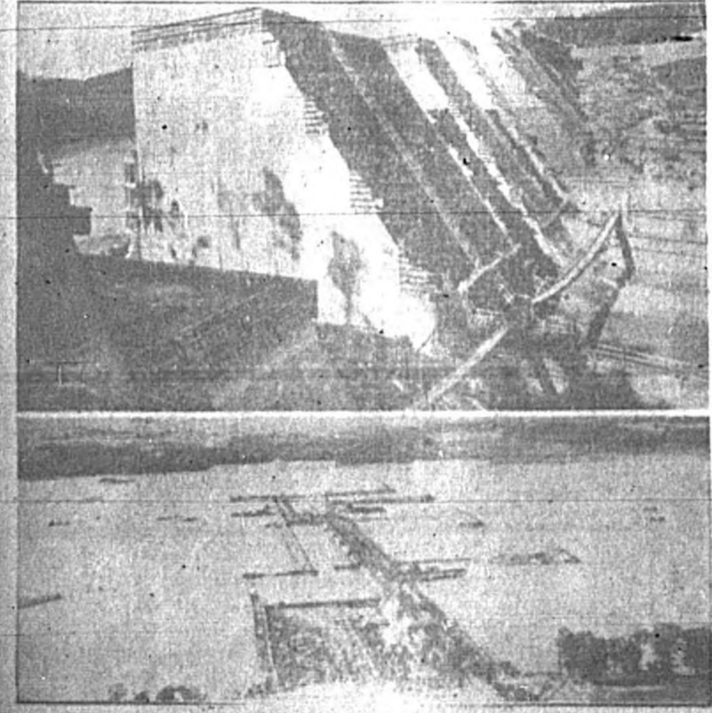
While Congress debates whether to enlarge the Tennessee Valley Authority's scope of operations, TVA construction moves ahead on its various fronts. At the top is a close-up view of a section of the $63,000,000 Norris dam...
