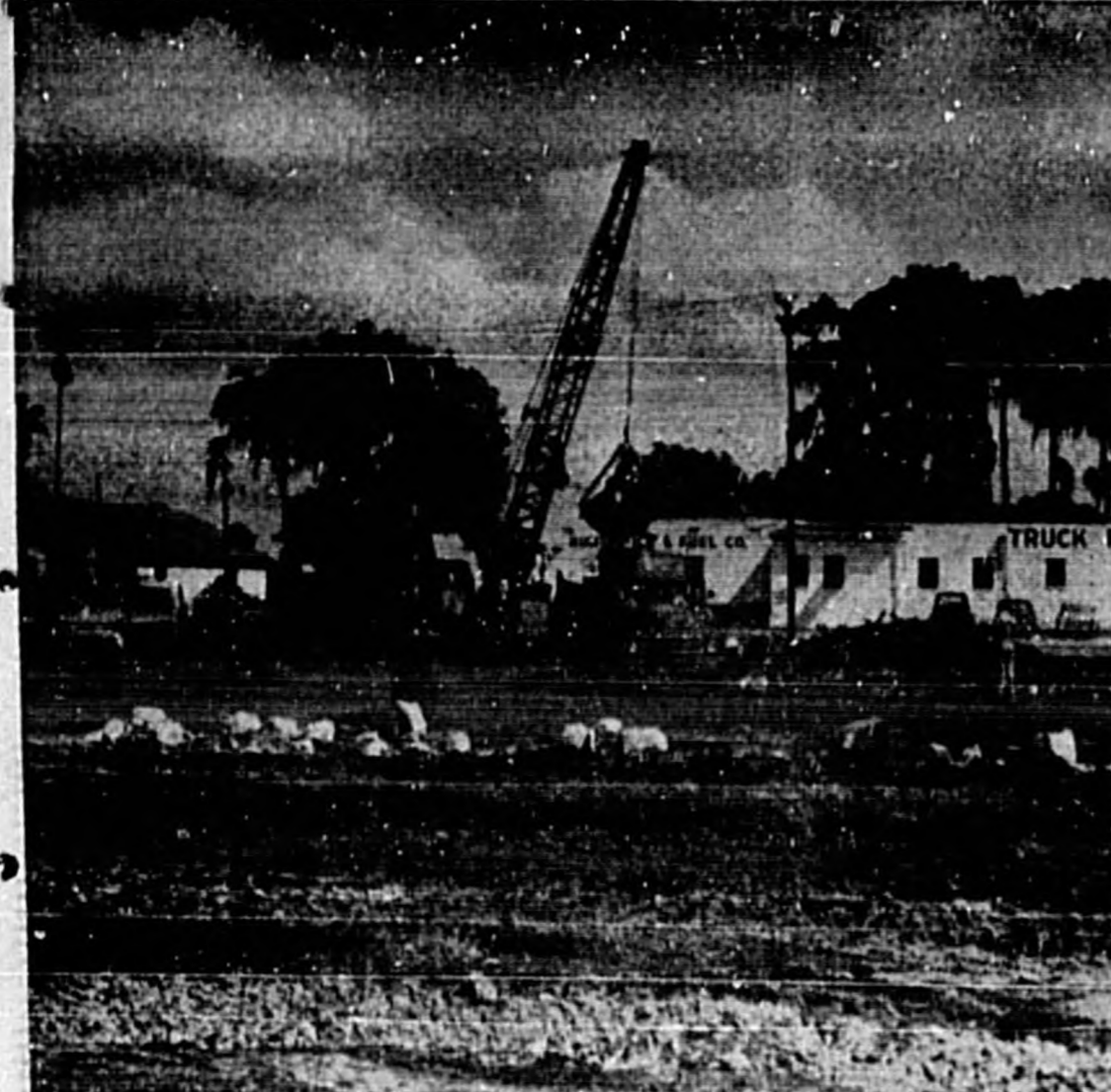
DEBRIS IS BEING CLEARED from the Sanford State Farmers' Market site with a full crew of workmen and mechanical equipment busy making ready for the rebuilding of a modern market. (Photo by Bergstrom)
