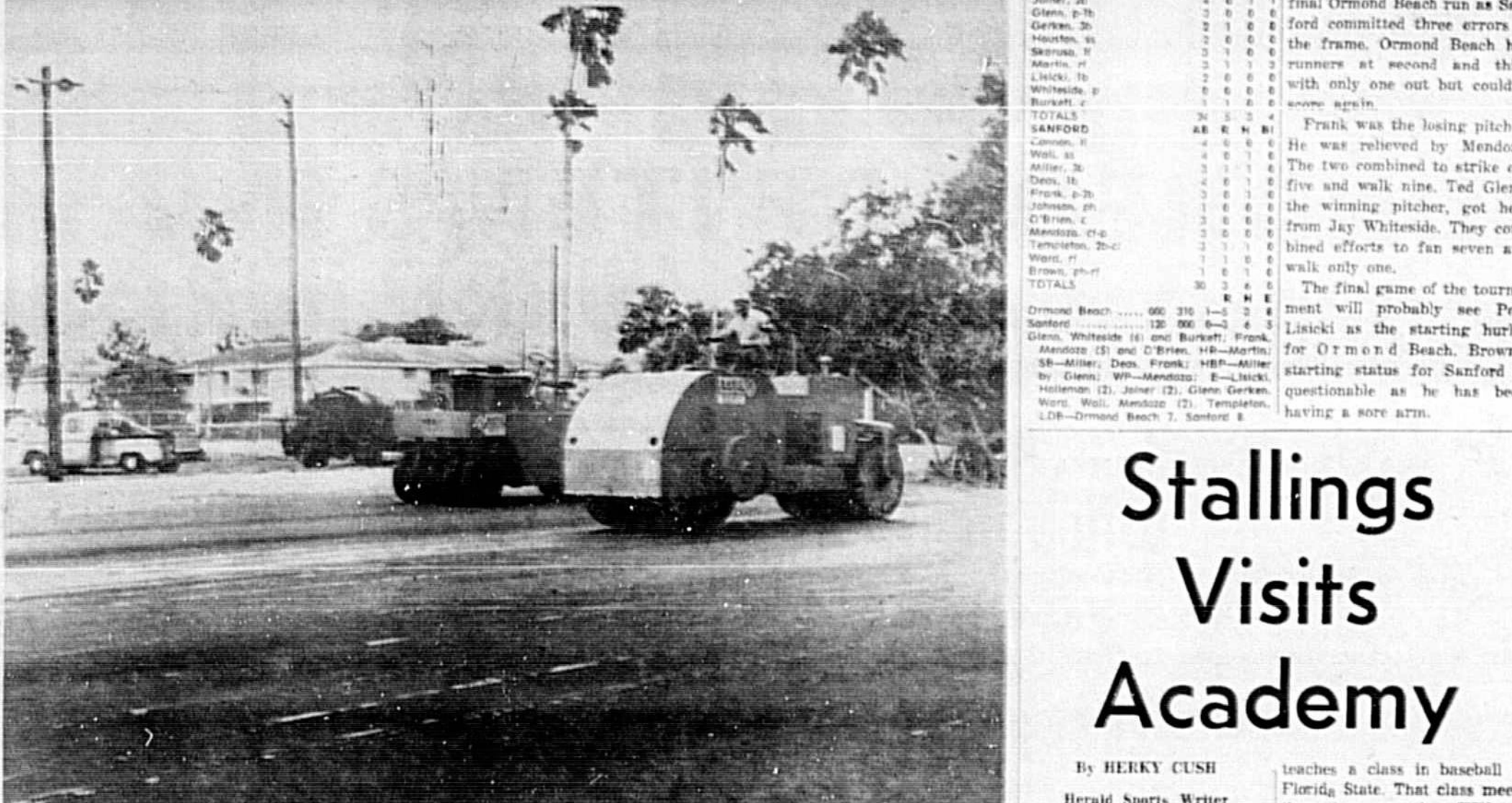
THE FINAL phase of the resurfacing of the tennis court complex began yesterday at Ft. Mellon Park. The courts are expected to be completed by August 1.
