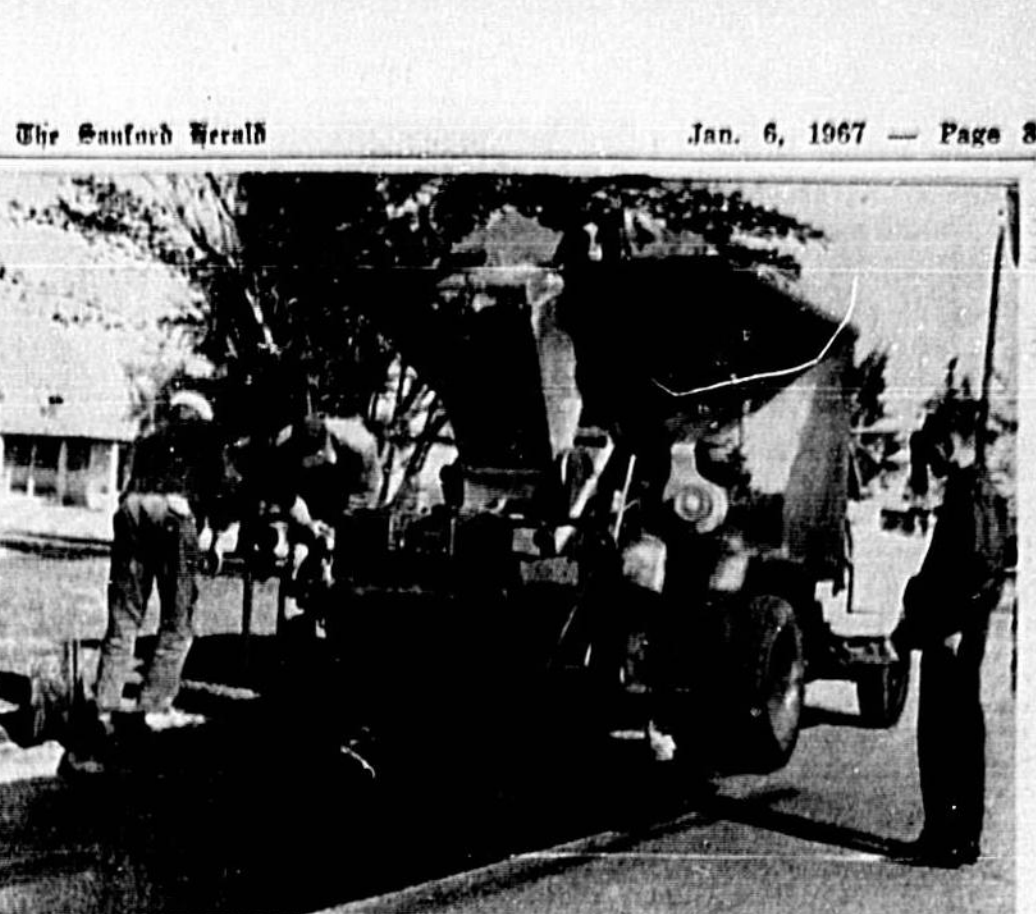
CITY WORK crews yesterday started work on resurfacing some five miles of streets as Sanford's resurfacing program got underway...
