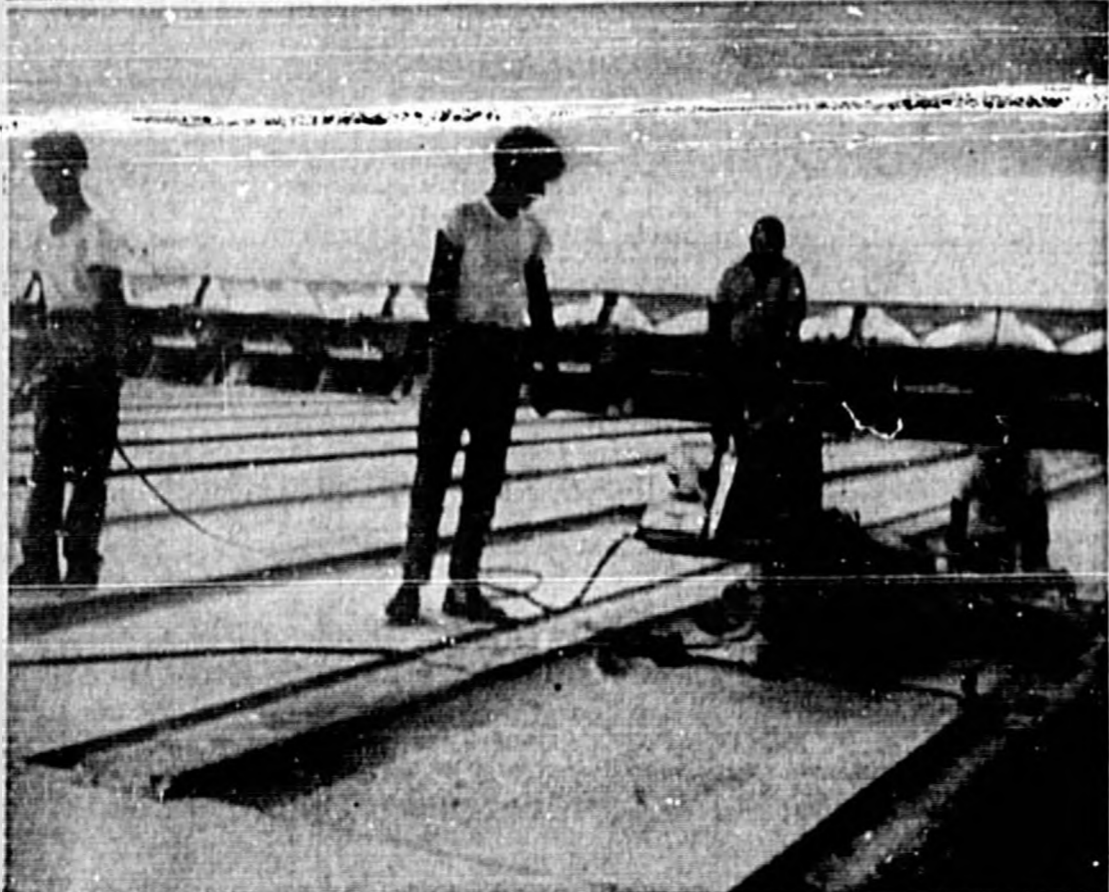
SKILLED TECHNICIANS put the finishing touches on resurfacing the lanes at Jet Lanes. The men applied many coats of paint to the lanes. According to ABC rules, the lanes now are cleared for two years before it is required to resurface them again.
