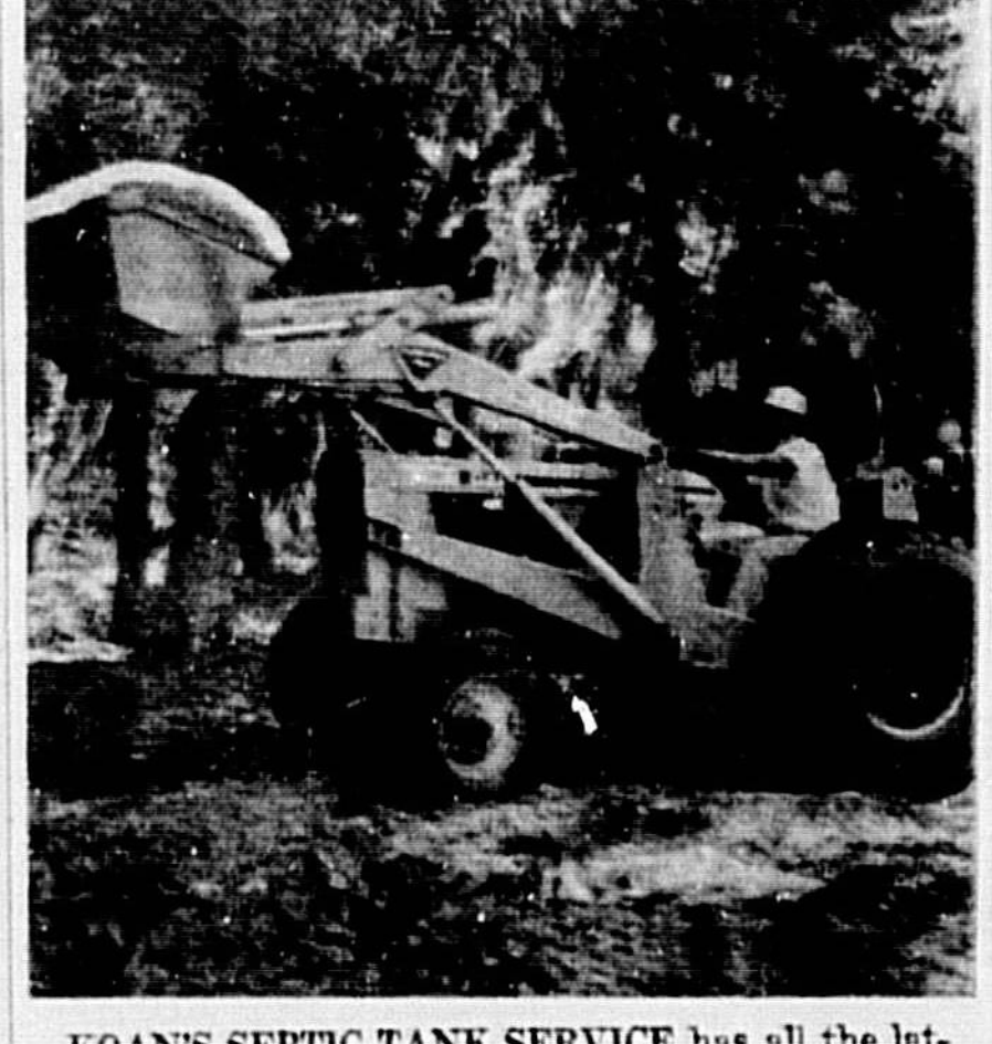
KOAN'S SEPTIC TANK SERVICE has all the latest equipment to serve your needs. Call Koan's at 322-5462 to have any question about your septic tank needs answered. Show here is one of Koan's newest pieces of equipment.
