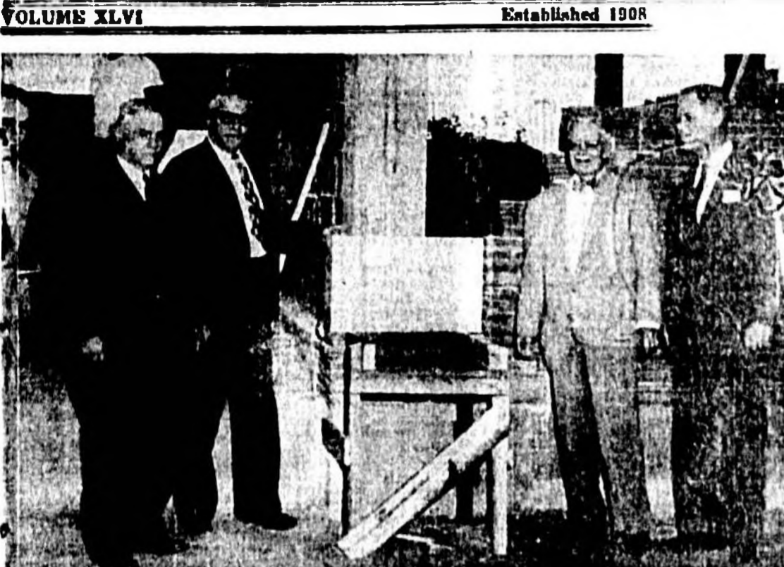
CORNERSTONE LAYING —Participating in the laying of the cornerstone yesterday at the Seminole Memorial Hospital were (left to right) Otis Fouraker, chairman of the board of County commissioners; Randall Chase, chairman of the board of directors, Fernald-Laughton Memorial Hospital; Francis Whitehair, chairman of the board of trustees of the Bert Fish estate; Dr. J. C. Boyce, president of the Seminole County Medical Assn., and T. E. Tucker, chairman of the board of trustees of the new hospital. (Staff Photo)
