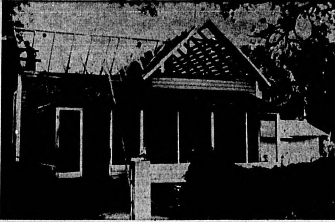
ANOTHER ENTERPRISE landmark, "The Old Burns House," which was built by Mr. and Mrs. W. J. Burns in 1906, is on the way down to be replaced by the new home of Mrs. Bertha Burns Hardin and Miss Sarah Burns.
