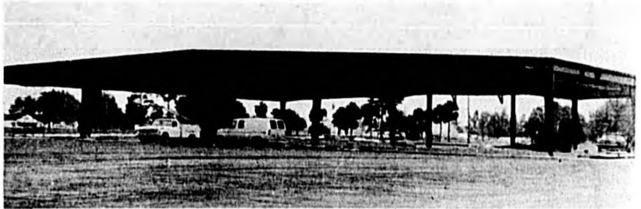
The 36,000-square-foot facility began construction Oct. 1 and is expected to be completed Feb. 2.
