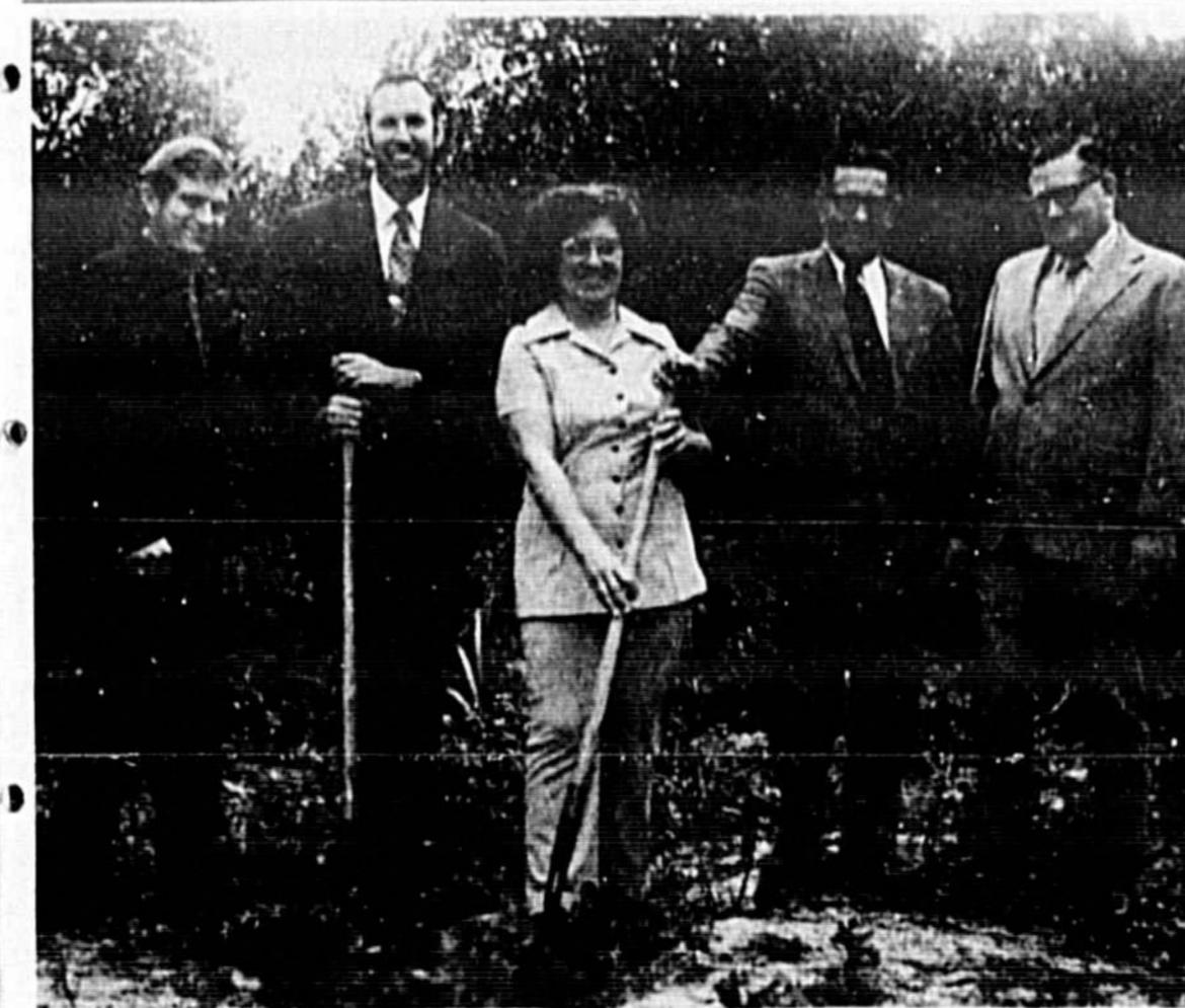
OFFICERS of the Mullet Lake Water Association are pictured as they prepare to break ground for the well which will be servicing 121 persons; (from left to right) William R. Holmes from the firm of Clark, Dietz and Associates, professional engineers; Ron Taylor, vice president, Mullet Lake Water Association; Ellene Bowen, secretary; L. M. Phillips, president and Ramon D. McGough, FHA representative. (Liz Mathieux Photo)
