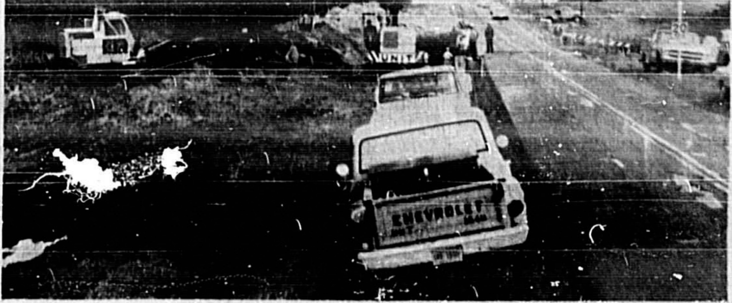
CLEARING of the right-of-way for construction of a new State Road 46 has been started at the Wokiva River (west) end of the five-mile project which will result in nine months in a two-lane highway on a four-lane right-of-way replacing the present SR 46. The project will cost $886,000.
