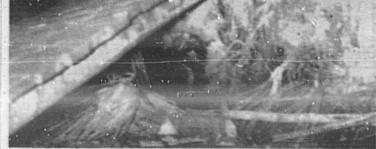
WALKING BRIDGE and tree undermined by heavy rains, bridge spans across ditch at the Joe B. McCawley residence on Wekiva River. McCawley reports that after most heavy rains the Wekiva River Road washes out around the culvert that runs under the road and in the process has at least three times undermined his home. The last heavy rains caused damage to his walking bridge. He states he has offered the County 10 feet of his land so they can maintain the deep ditch to stop this undermining to his property. (Liza Baker Photo)
