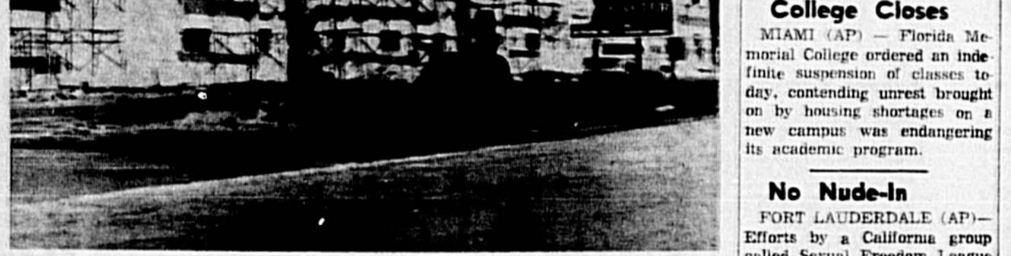
NEARING COMPLETION is this large apartment complex to be known as Fern Park Apartments. Located on Oxford Road across from English Estates School, the one and two bedroom apartments are being built by Stewart and Poole, developers. They will feature a pool, playground and day nursery. (Photo by Jane Casselberry)
