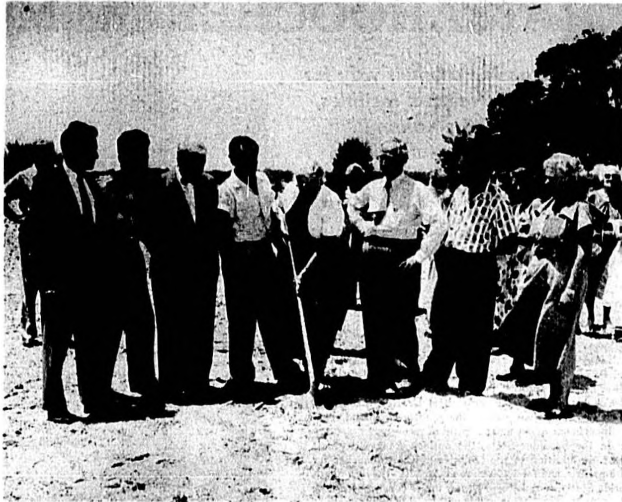
IT WAS with confident minds and over-joyed hearts that the Little Theatre members, officers, and interested outsiders of the community gathered to break ground for the building which is now all that any Little Theatre group could want.
