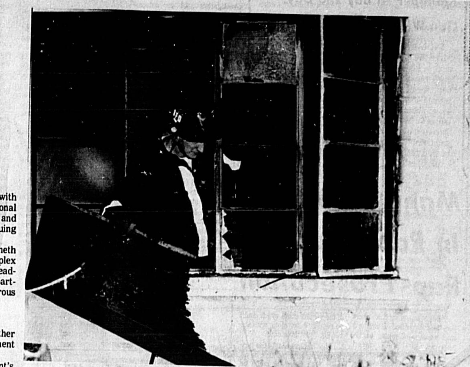
FIRE DAMAGES SANFORD HOME Sanford Fireman Bill Price removes burned material from Jerry Walker residence at 516 E. Fifth Street after blaze which occurred Tuesday. One person reportedly was slightly injured in the blaze. Cause of the fire was not immediately determined. Another fire, in Midway, resulted in a fatality Tuesday night. Details in Action Reports, Page 2-A.
