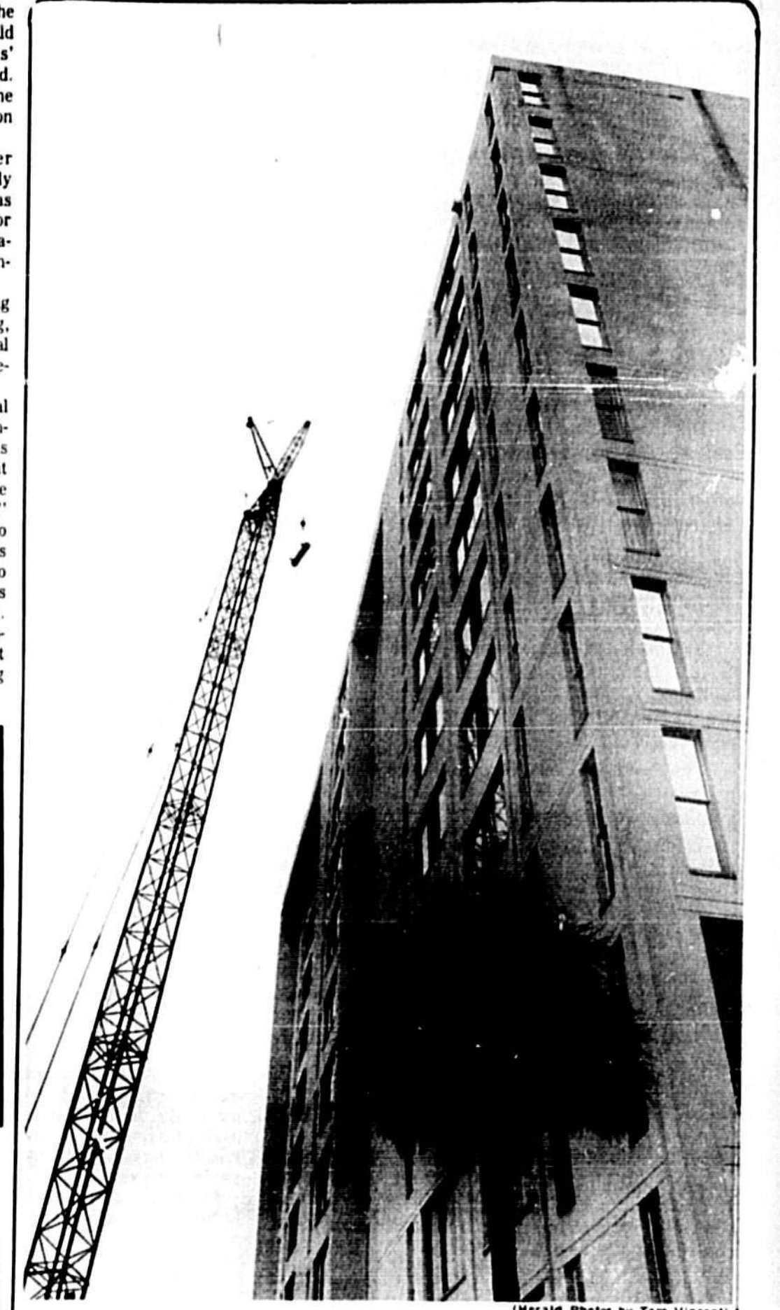
A crane lifts a new air-conditioner compressor to the roof of the 12-story Bram Towers in downtown Sanford, Fla. Arlene Boyd, manager of the senior citizen retirement center, said the crane had to be used because the compressor is too big to fit in the elevator.
