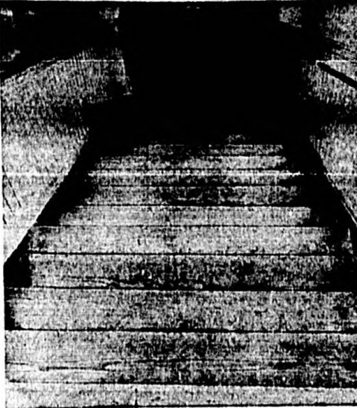
IF YOU VOTE for the School Bond Issue you will help eliminate such hazardous conditions as this one at Sanford Grammar School. Steep, wooden stairs are dangerous anywhere, but more so in a school where children constantly use them. (Photo by Bergstrom)
