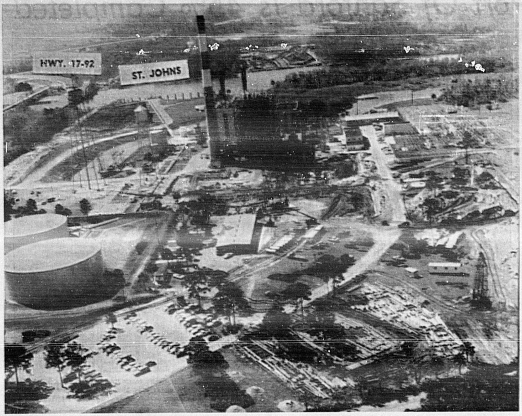
CONSTRUCTION is underway on the $40 million conventional power plant of Florida Power and Light Company on its present plant site on the St. Johns River. Manager Scott Burns reported 160 construction men are now employed on the job by Mid-Valley Contractors, and the payroll will jump to 300. (Aerial Photo by Bill Vincent Jr.)
