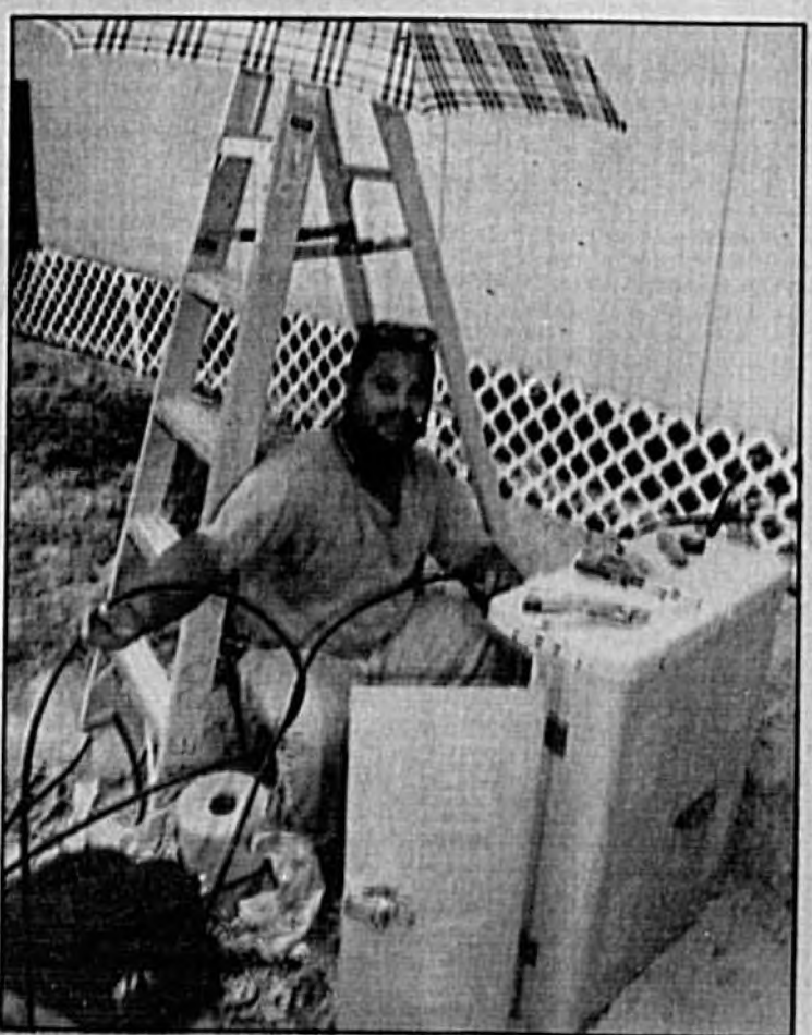
Edward Febres, a cable splicer for Hincfels and McCoy's Telecommunications of Ocoee, splices cable and fiber optics lines outside of Midway Elementary school while his large umbrella keeps the sun off of him.
