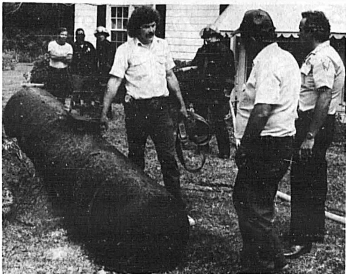
With the tank out of the ground, Ron Coe, left, George Bumgardner, and Mike Hoening discuss loading it on trailer
