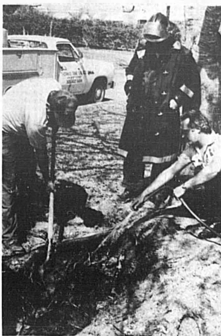
Sanford Fireman Fred Bowen watches as George Bumgardner, gas company employee, digs around the tank and fireman Mike Hoening operates hose.
