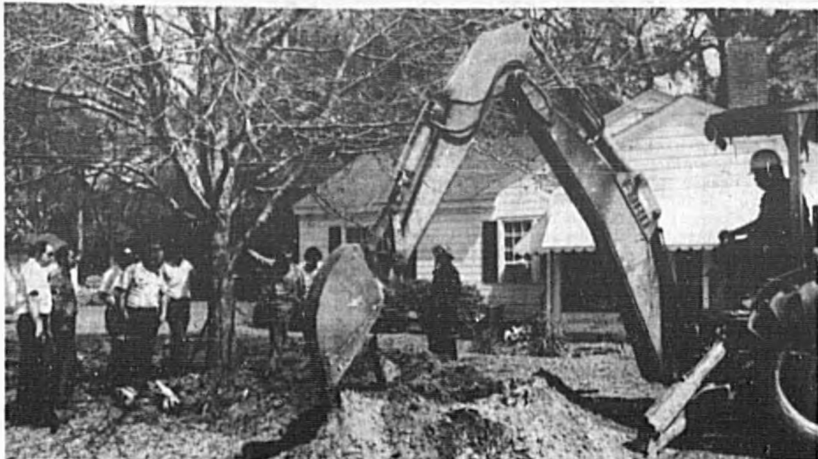
City's backhoe called in to dig dirt and roots away from tank.
