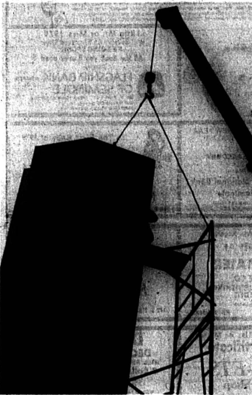
AND DOWN IT GOES Solid concrete column cracked near the base by the Christmas Eve windstorm was removed late Wednesday from the front entrance of Casselberry City Hall by B&B Steel Erectors of Orlando for $675. Although apparently undamaged, a matching column will be removed on Friday. "It was a matter of safety," said City Clerk Mary Hawthorne. "We didn't want it falling on someone." The council will decide later what to do about rebuilding the entrance.
