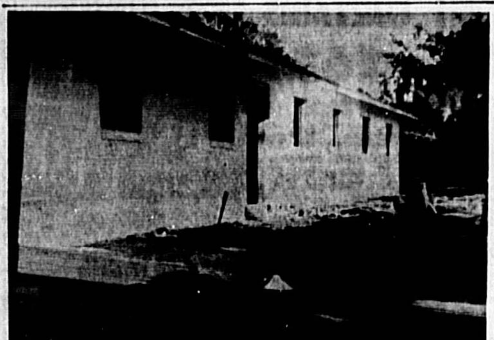
CONSTRUCTION on new educational wing of First Baptist Church of Geneva is progressing on schedule. The new unit, being built at an estimated cost of $15,000, will have two nurseries, departments for beginners, primaries, and intermediates, an assembly hall which can be converted into a banquet hall, a kitchen, and storage facilities for air conditioning and heating. (Herald Photo)
