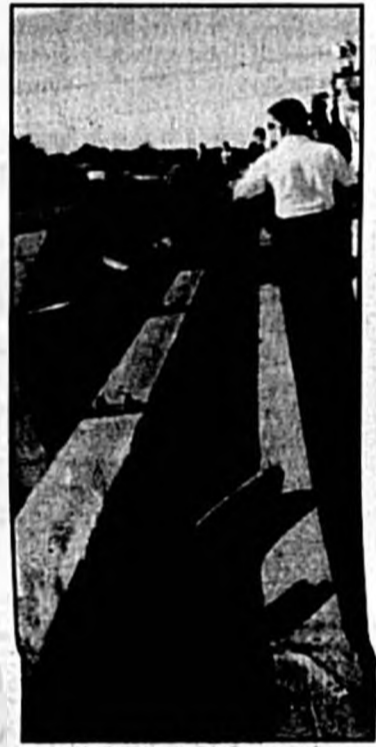
Photo submitted by Travis Hamilton. An SUV dangles Wednesday from the Interstate 4 bridge over State Road 46. A thin bolt was the only thing that kept the vehicle from falling to the road below.
