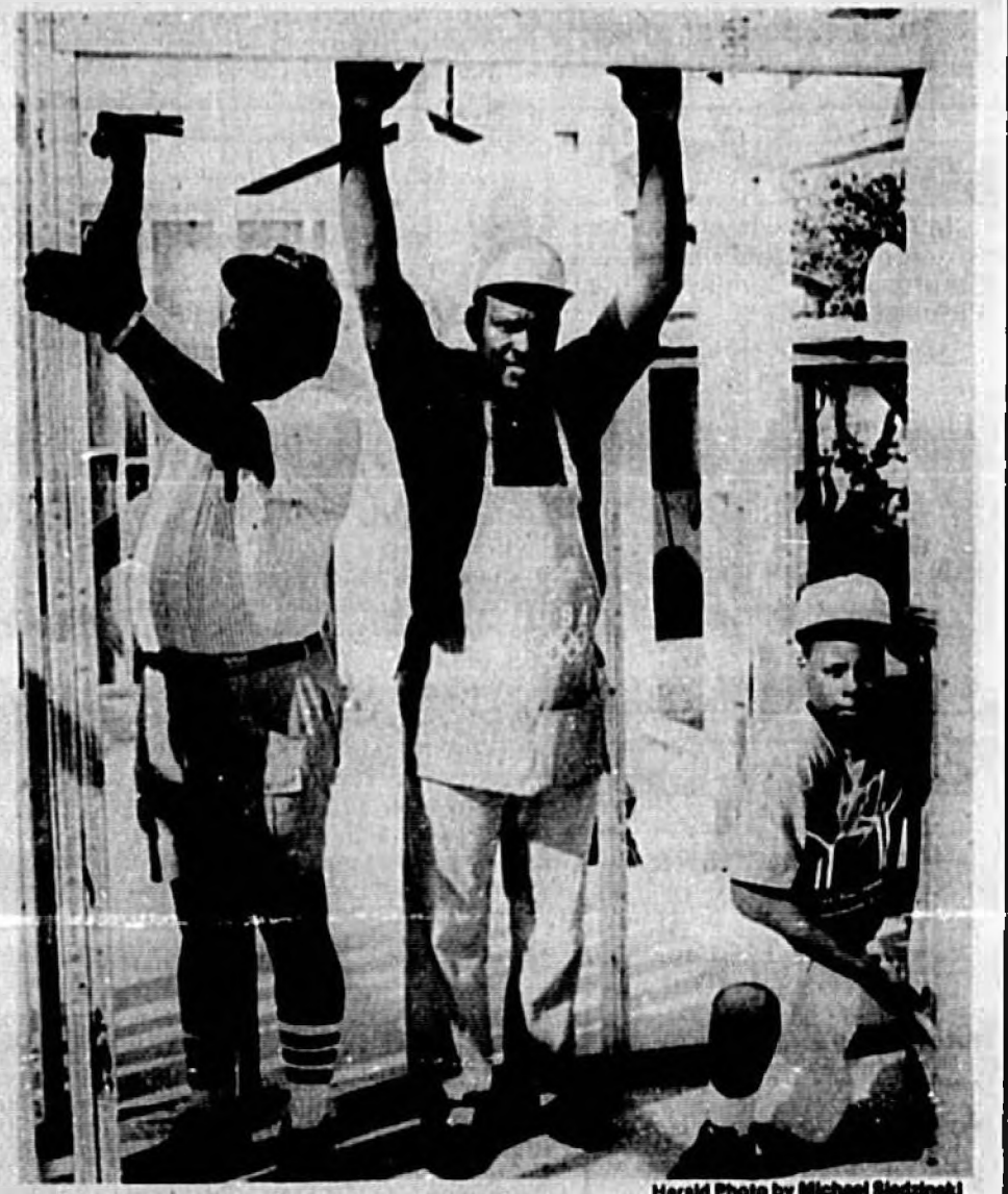
Holding on to his own home, Robert Johnson, center, rests for a moment while Lambert Mills and Johnson's son Robert Jr. continue to work on the Johnson house.
