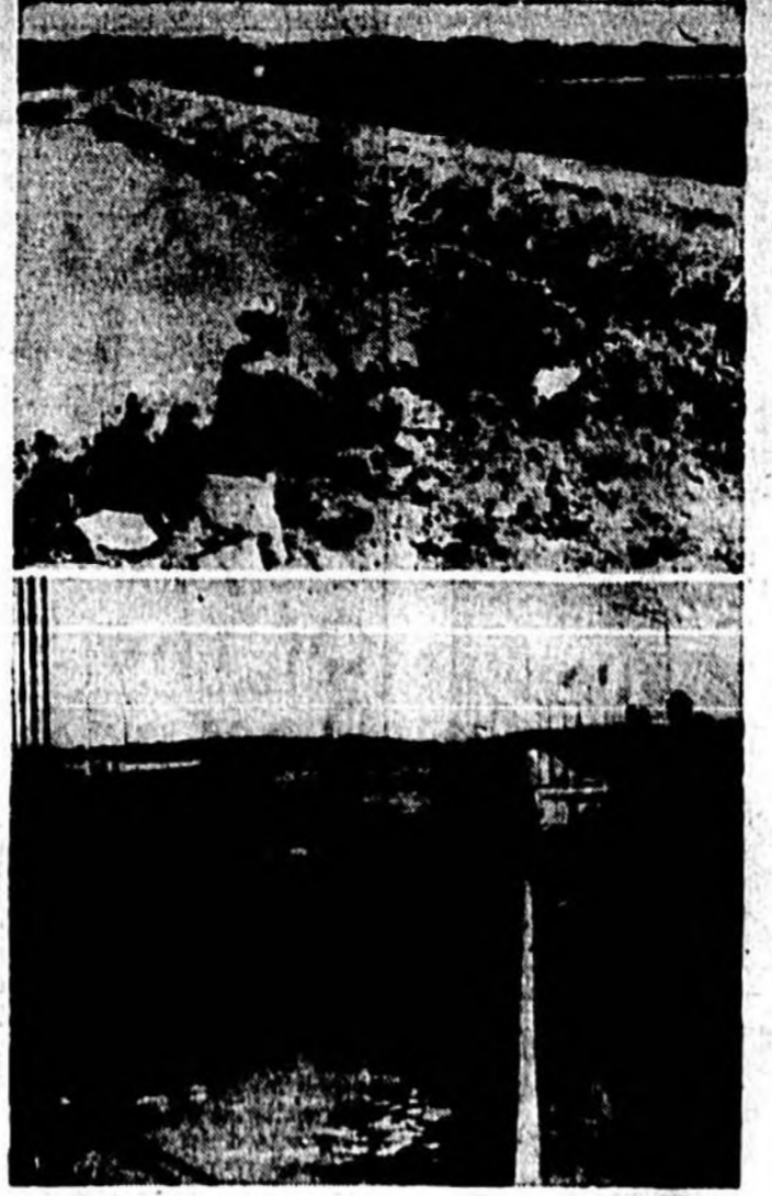
DYNAMITE TO OPEN SEAWAY CANAL —Dave Forrester, 67, keeps a watch over the dynamite-seeded temporary dam (top) that holds back waters of the St. Lawrence River at Massena, N. Y. Destruction of the dam will flood the new Willgoose-Spenser Canal (bottom) of the St. Lawrence Seaway with 27 feet of water. Standing at the Dwight D. Eisenhower lock are Rear Adm. Heber M. McLean (left), who will direct Seaway operation, and Capt. J. J. Strokiak, chief dispatcher for the canal.
