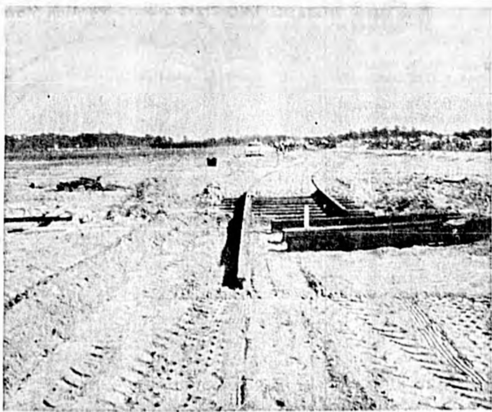
RAILROAD SPUR nearly completed into the Hunt plant from the ACL tracks on the site of the new vegetable processing plant.
