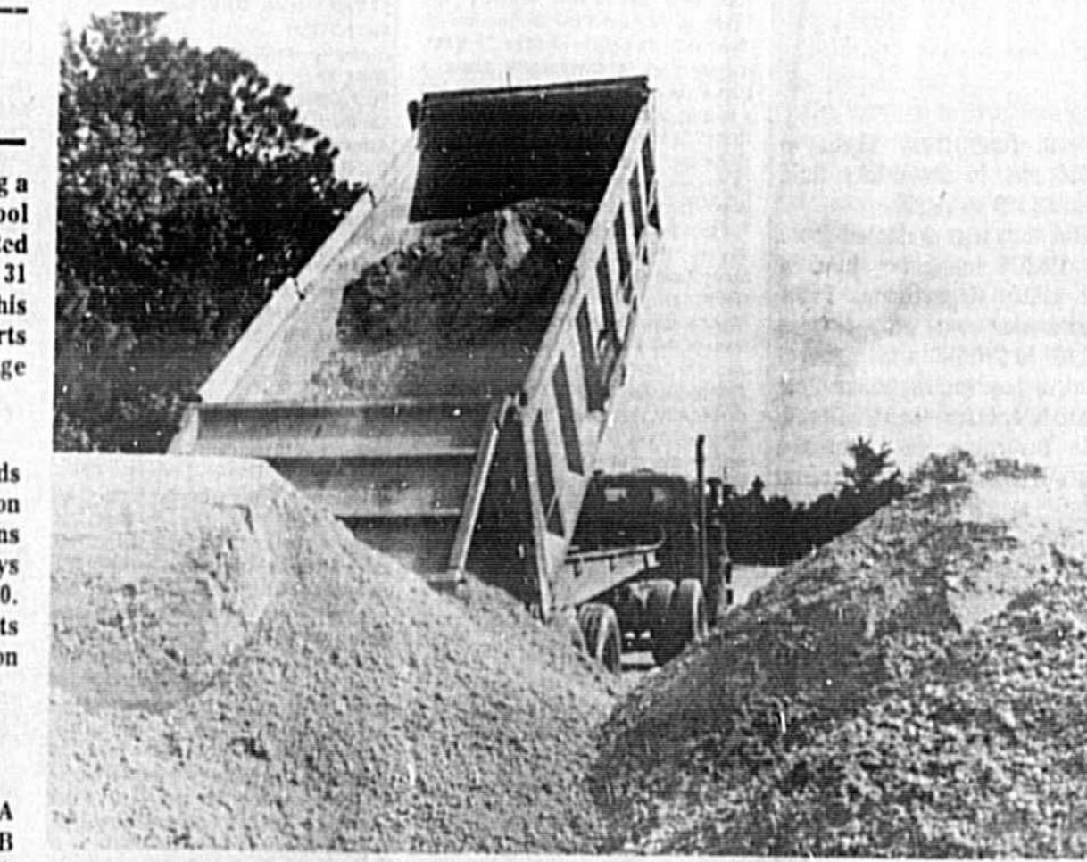
ZOO PAVING STEP CLOSER Paving of the roadways at the new Central Florida Zoo moved one step closer Wednesday when heavy dump trucks moved 40 loads (1,000 tons) of time rock into the area to be paved. The new zoo is located off U.S. 17-92 and Interstate 4 north of Sanford. (Herald Photo by Bill Vincent Jr.)
