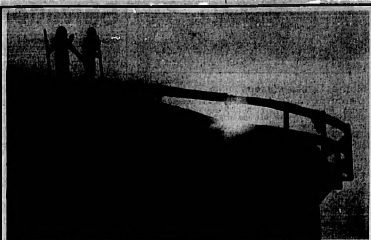
Dawn workers Two construction employees this morning work at the Sanford wastewater treatment plant on Poplar Avenue as the sun rises behind them. The construction project at the site is part of the city of Sanford's effort to upgrade the quality of treated sewage so that it may be used as reclaimed water for irrigation. Herald Photo by Tommy Vincent
