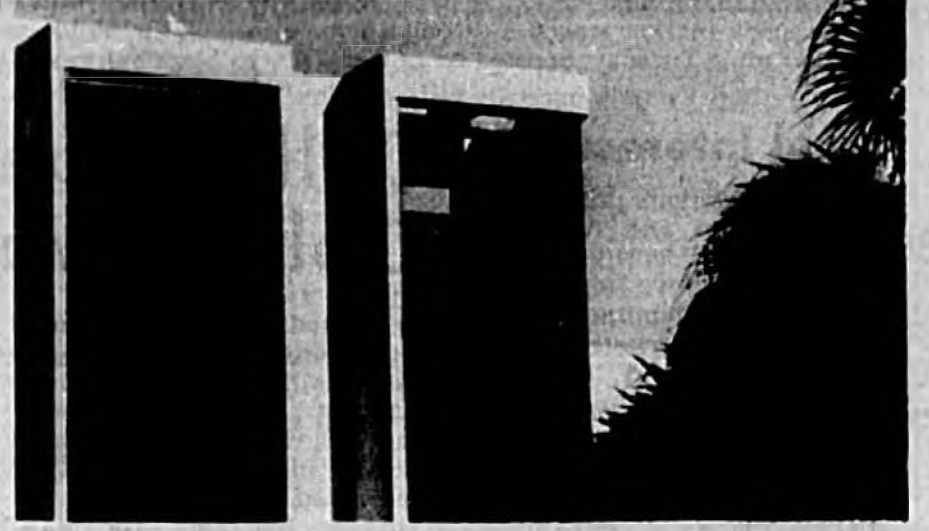
Seminole County will have to replace a 60- by 80-inch exterior glass window that shattered this week on the north east corner of the county courthouse. Courthouse employees were startled when its hundreds of coin-sized pieces plummeted four floors, bouncing off interior windows and frame work. It is the third window to break since the building was built in the 1970s.
