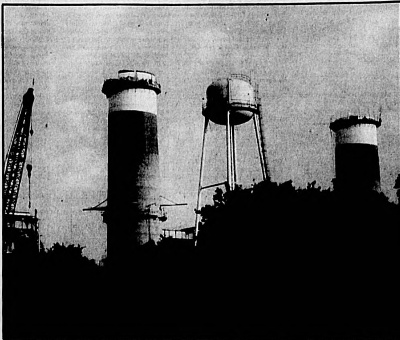
The old FP&L smokestacks are on their way down after years as a landmark for travelers along 17-92 and Interstate 4. The stacks are no longer needed as the power plant recently completed a change to natural gas — a cleaner burning fuel than oil.
