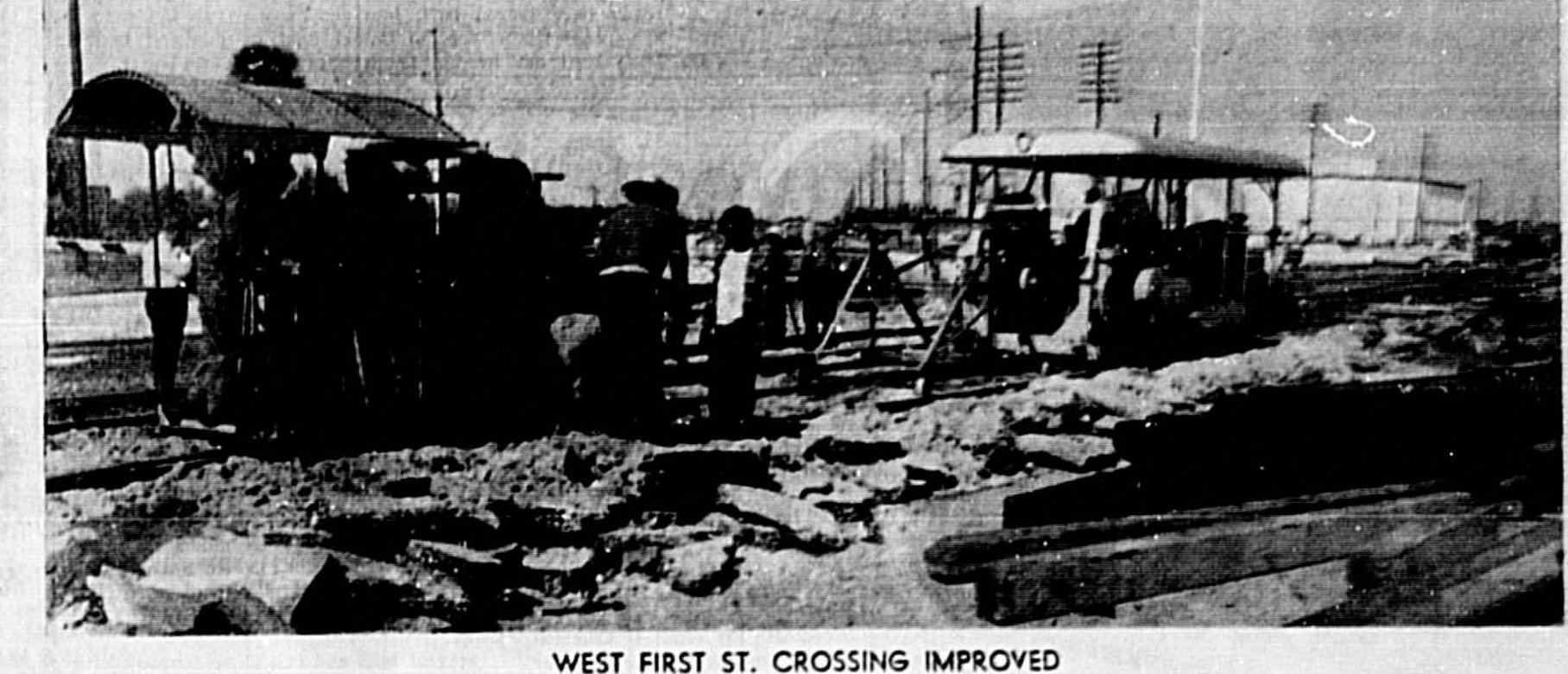
WEST FIRST ST. CROSSING IMPROVED New paving is being laid at the SCL crossing on West First Street. SCL crews are pictured tearing out the old road bed between the rails. One-lane auto traffic prevails during the repair work.
