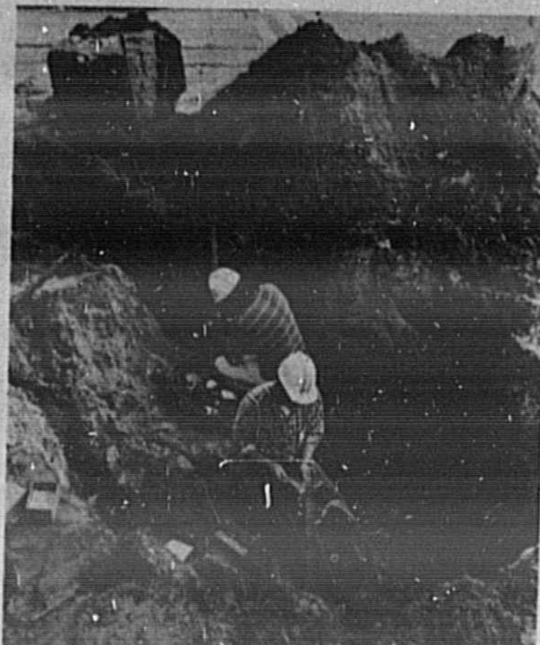
TELEPHONE CABLE CUT
