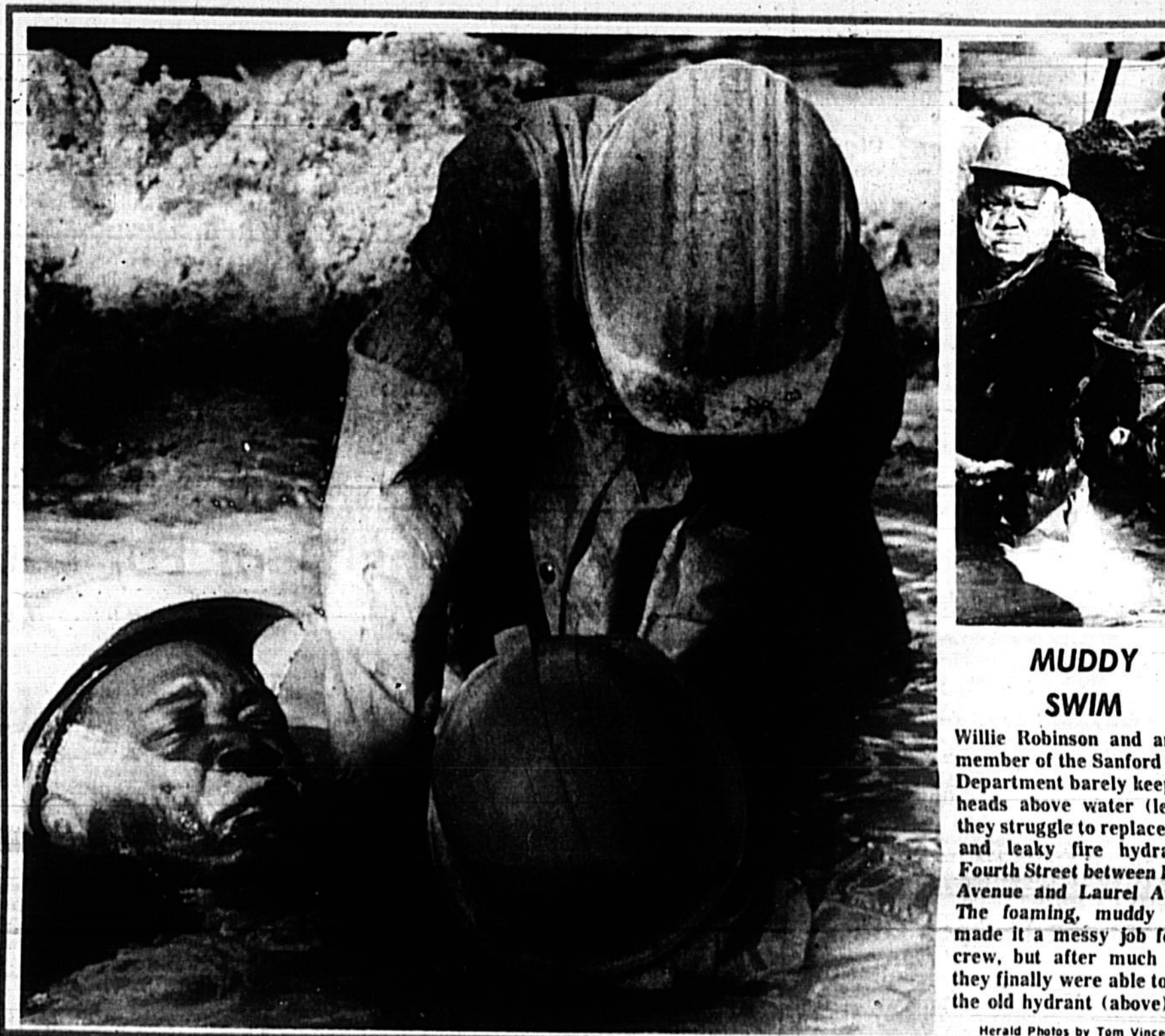
MUDDY SWIM Willie Robinson and another member of the Sanford Water Department barely keep their heads above water (left) as they struggle to replace an old and leaky fire hydrant on Fourth Street between French Avenue and Laurel Avenue.
