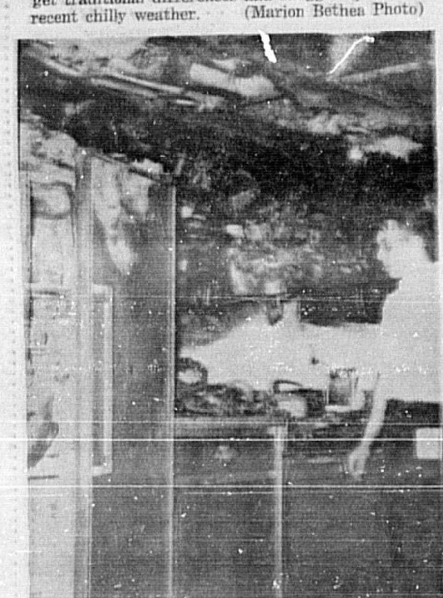
EXTENSIVE damage to the home of Mr. and Mrs. Kenneth Moore, Spring Valley, resulted from a forgotten burner under a frying pan, according to Forest City Volunteer Fire Department. Fireman Robert Clark surveys the damage. (Maryann Miles Photo)
