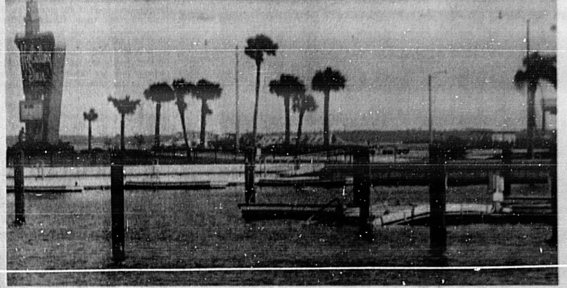
High Winds Sink Floating Pier SIX-FOOT-WAVES last week caused the western end of the floating pier at Monroe Harbour Marina, on Sanford's lakefront, to sink. The hollow concrete blocks filled with water during the wind-storm, causing the floats to sink. Manufacturer's agents are coming to Sanford to inspect the damage. (Staff Photo by Don Vincent)
