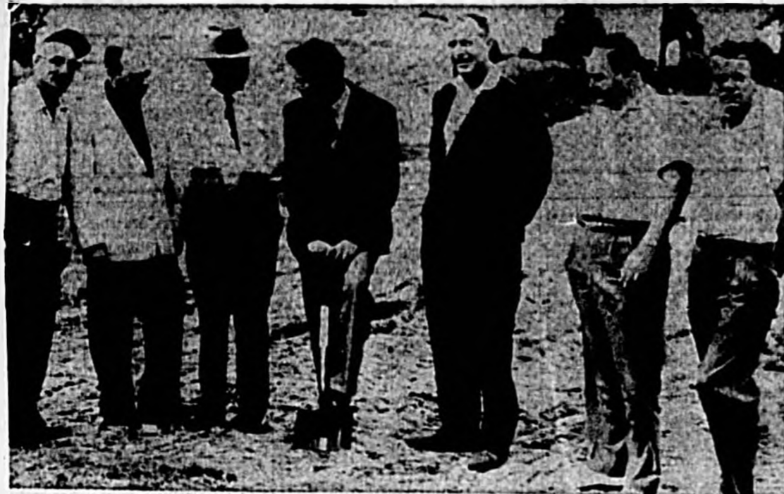
CONSTRUCTION IS STARTED on the Goldboro Swimming Pool when Mayor David Gatchel turns the first spadeful of dirt to get the project underway. At the brief ceremonies this morning were (left to right) City Commissioner Merle Warner, A. L. Wilson and Earl Higginbotham, Mayor David Gatchel, Commissioner F. D. Scott, Architect John Hurton IV, and Leroy Robb representing Carroll-Daniel Construction Co. to whom the contract was awarded. (Photo by Bergstrom)
