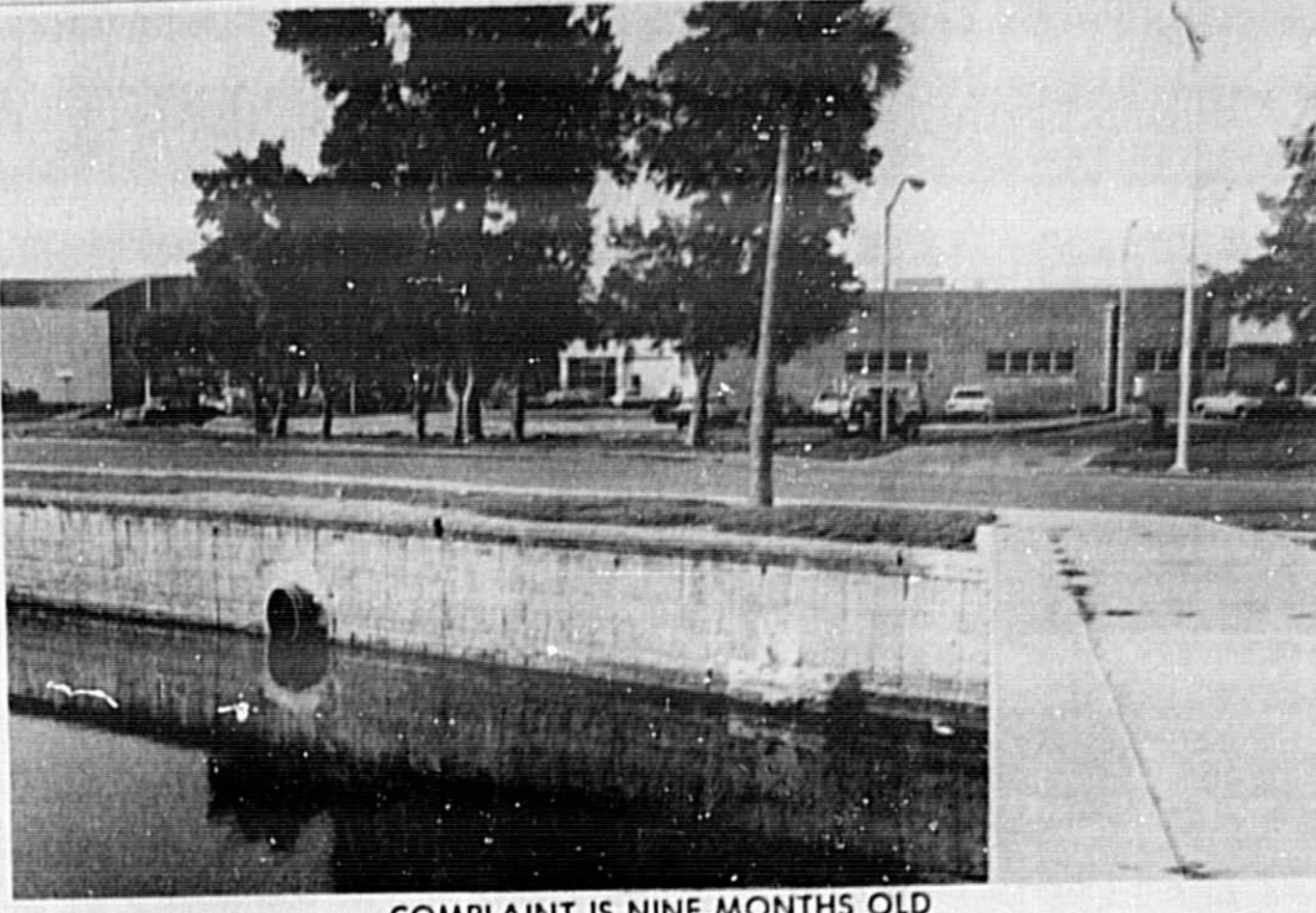
COMPLAINT IS NINE MONTHS OLD The photograph was published nine months ago by The Sanford Herald when Sidney Vihlen Jr. first called attention to untreated sanitary waste flowing through this storm sewer into the City of Sanford harbor across from the post office. He has renewed his request the City be compelled to eliminate the situation (see accompanying article by Jane Casselberry).
