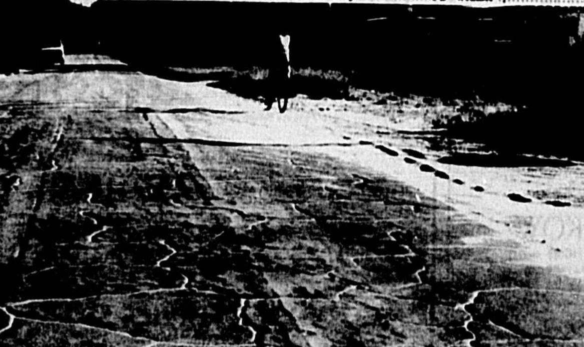
CRACKED ROADWAY ON SUMMERLIN AVENUE
