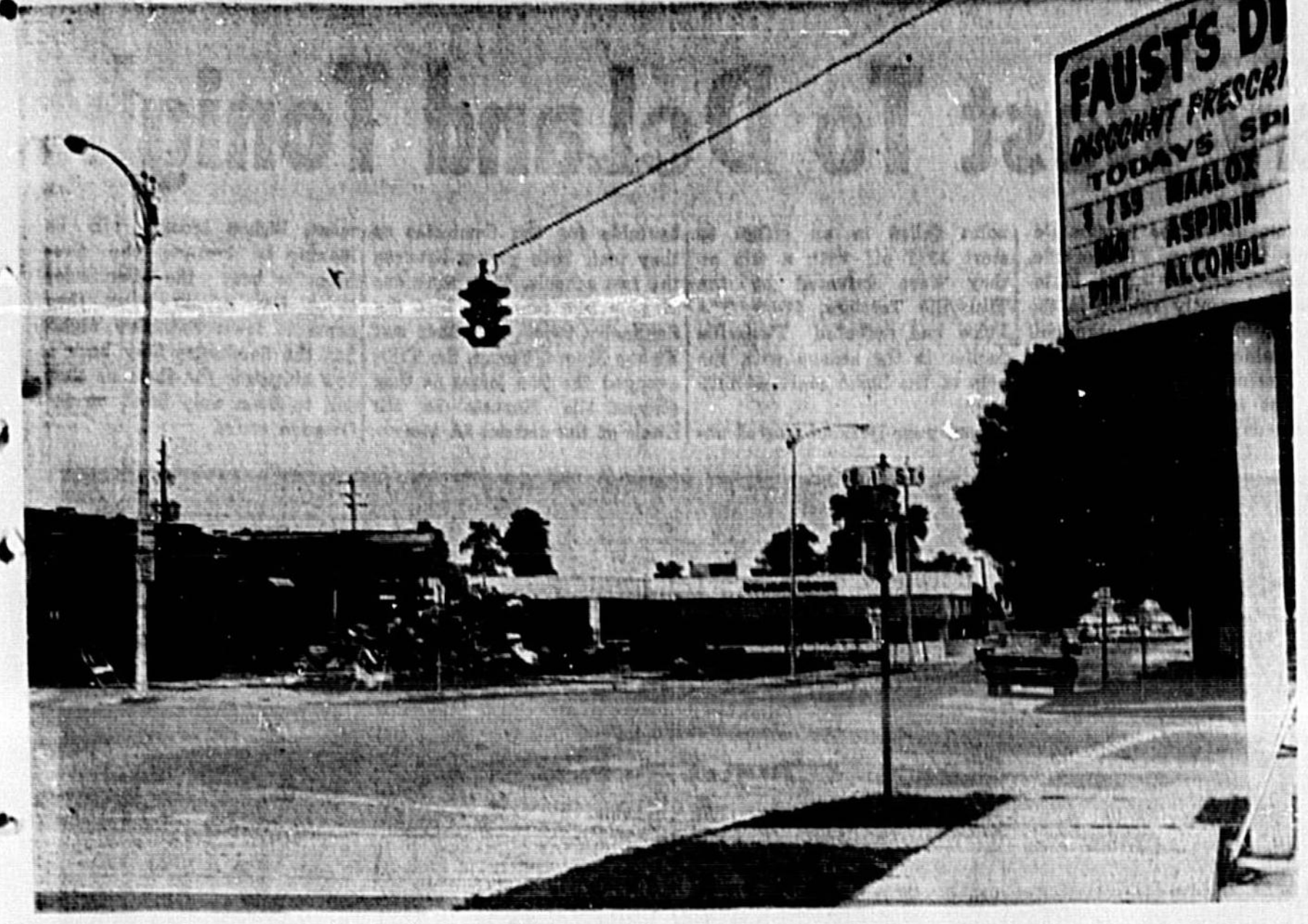
DEMOLITION continues on one of Sanford's former landmarks at the corner of East First Street and Sanford Avenue. (Photo by John A. Spolski)
