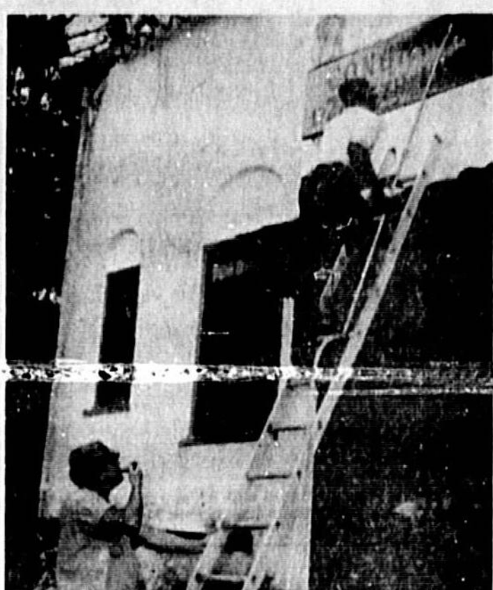
WASHING down the face of the Little Red School House in preparation for a paint job are Ed Sessions and Billy Range of Yensh Maintenance Service.
