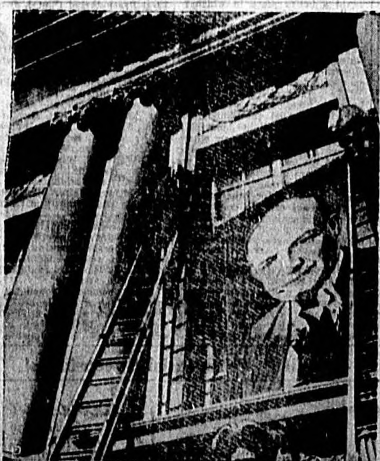
WORKMEN install a large picture of Gen. Dwight D. Eisenhower on the front of the Conrad Hilton Hotel in Chicago, headquarters for both Sen. Robert A. Taft and Gen. Eisenhower. (International Soundphoto)
