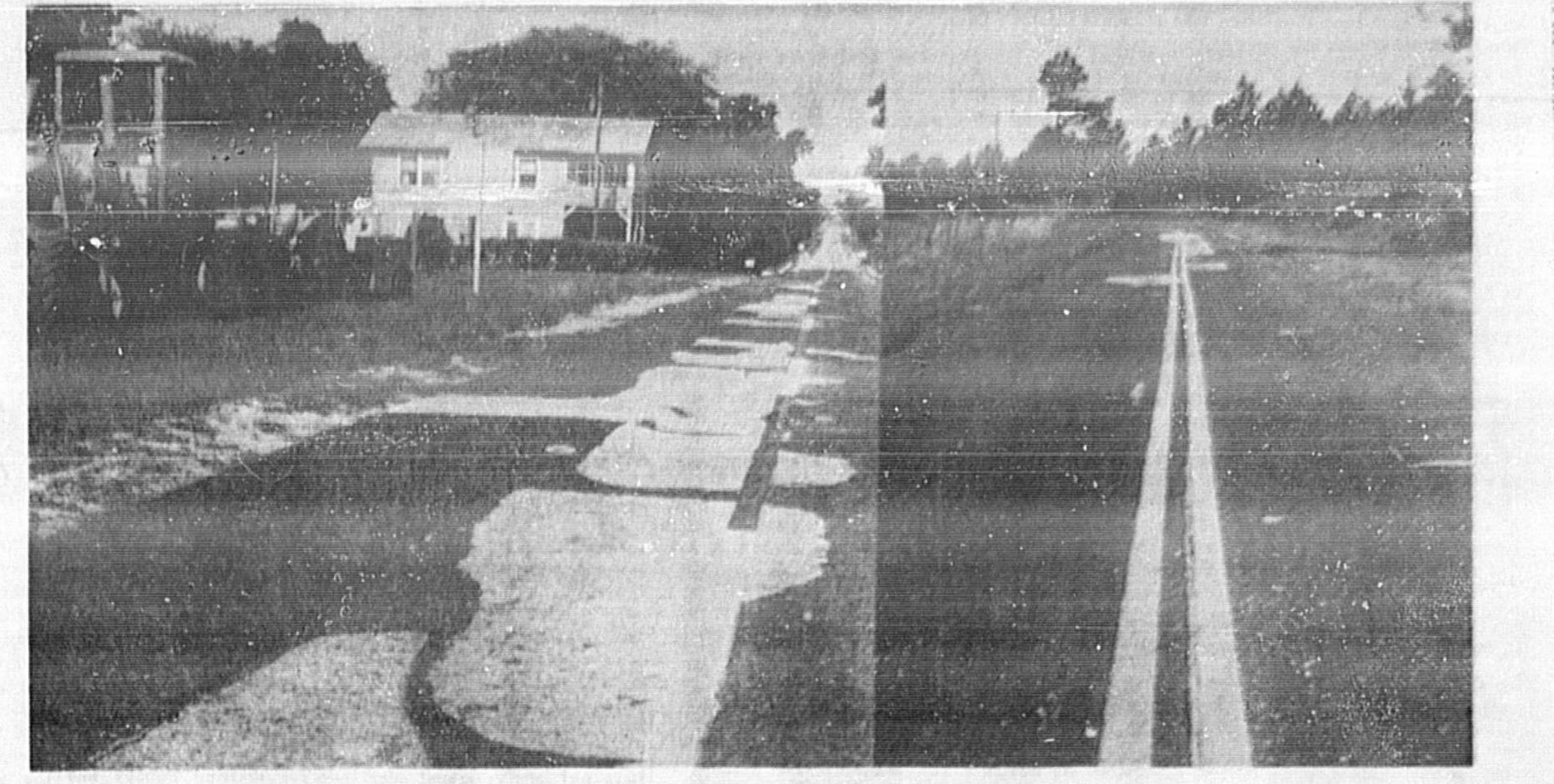
SHOW WINDOW? OR ... JUMPING TO CONCLUSIONS TEMPORARY REPAIRS, such as filling chuck holes, grading and rolling berm (note road machinery at left), painting new center lines (right photo), were underway on State Road 46 today by the State Department of Transportation.
