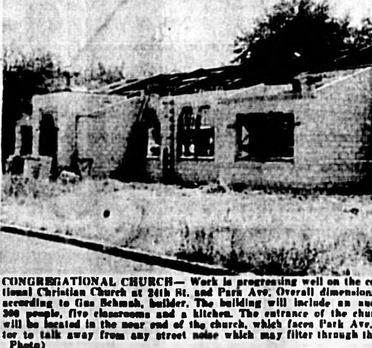
CONGREGATIONAL CHURCH—Work is progressing well on the construction of the new Congregational Church at 24th St. and Park Ave. Overall dimensions are 41 x 33...
