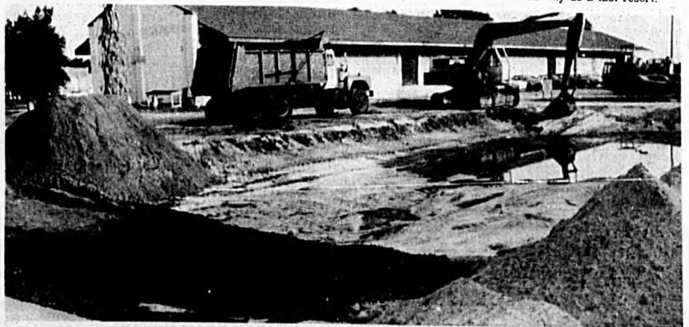
This is all that's left of the W. Atlee Burpee Seed Co. building, First Street, Sanford, where three men were killed Friday when a wall collapsed during demolition of the structure.
