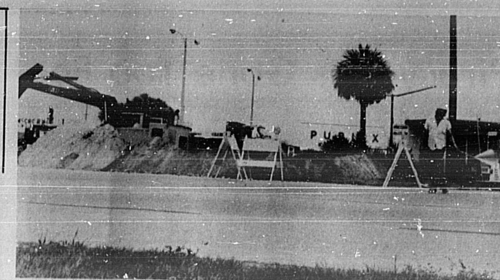
PREPARATION FOR 17-92 & 436 EXPANSION UNDERWAY CONDUIT is laid for telephone cable moved to make way for additional turn lane to be part of the $1.28 million improvements to begin construction next month. Work is expected to slow traffic at the busy Casselberry intersection for at least 10 months as additional lanes are built in both directions on 17-92 and 436.
