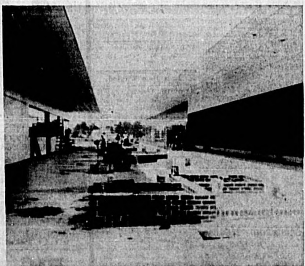
CONSTRUCTION on brick planters and concrete benches in the Shopping Mall at the Seminole Plaza Shopping Center, Hwy. 17-92 and SR 436, is well underway. Shrubbery and flowers will fill the planters and the entire area will be spotlit at night. (Herald Photo)
