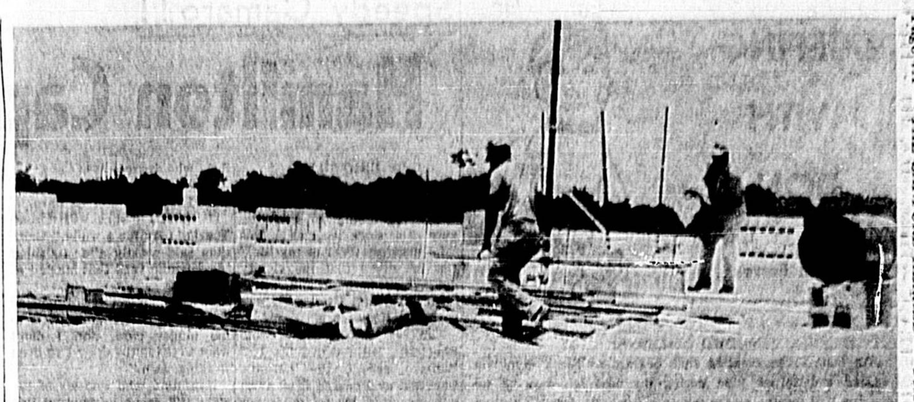
CONSTRUCTION has started on new facilities for Mr. Barney's School at Dodd Road and Howell Branch Road for housing 312 pupils. It is slated to be ready for opening day of school Sept. 2.
