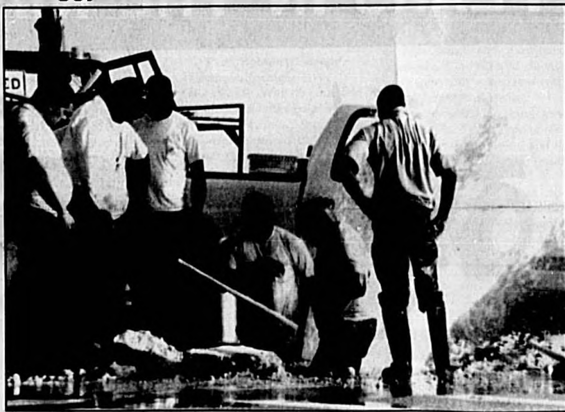
City of Sanford Utility Department workers repair a broken water main Wednesday afternoon. The break occurred at the intersection of 1st Street and Highway 17/92. The repairs took several hours, but the crews had the water main fixed by Wednesday evening.
