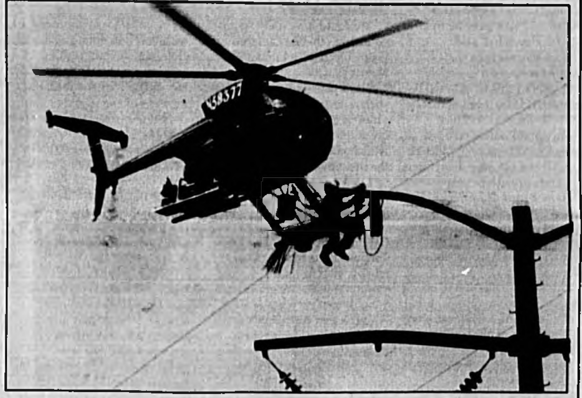
Hovering above Oaklawn Park Cemetery on Rinehart Road, aerial lineman Frank Dicks of Air2 Company of Miami installs pulleys on the power poles belonging to Florida Power Corp. The pulleys will be used to install fiber-optic lines on the poles.
