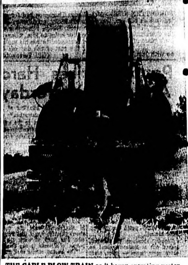
THE CABLE PLOVER TRAIN as it began operating yesterday in laying one leg of the Southern Bell Telephone Company cable between Ovido and Chuluota. The machine, operating at a top speed 10 to 12 miles per hour, digs a 30-inch deep ditch, lays the cable, and covers it up. All in one operation. (Photo by Bergstrom)
