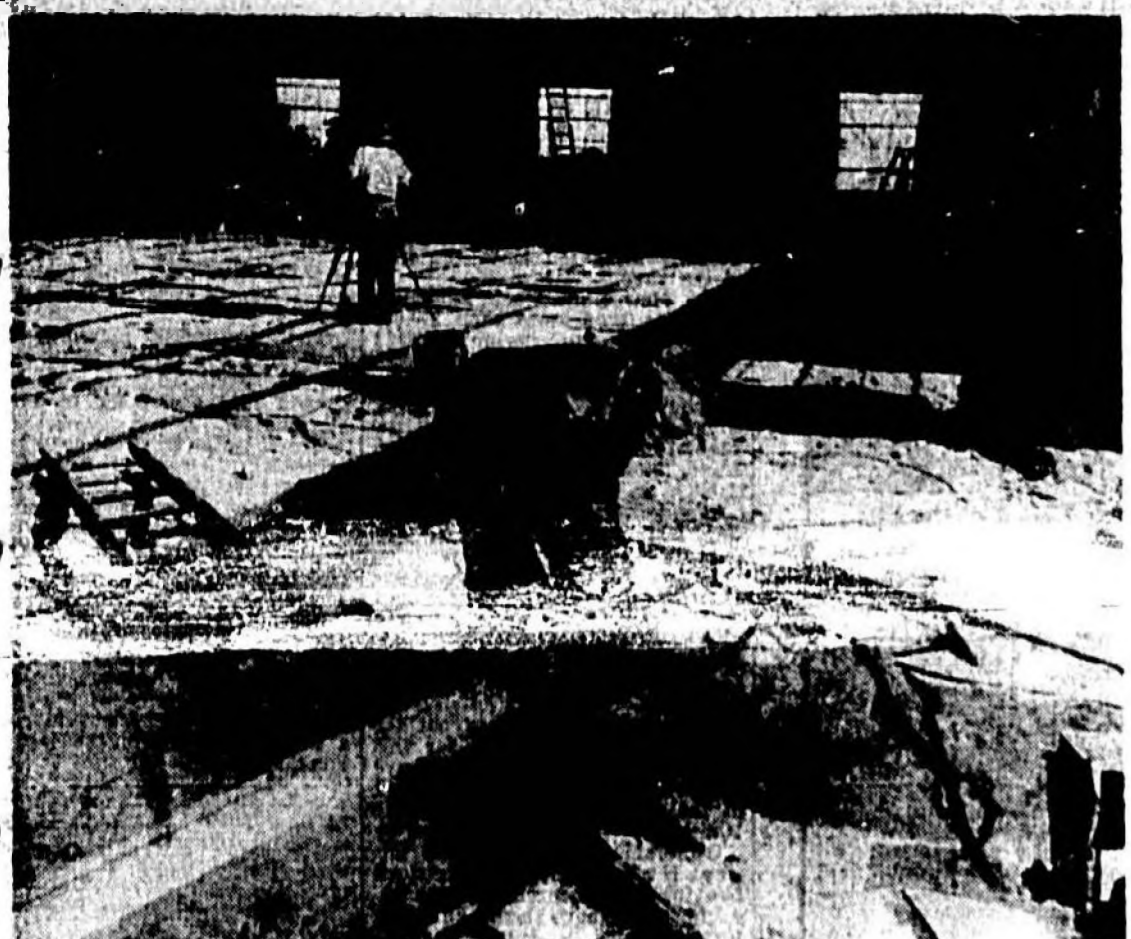
WORK IS PROGRESSING on the construction of the new warehouse building being built by the Southern Chemical Co. The interior of the building is shown in the picture. A workman with a cutting torch is in the foreground, and another workman with a transit in the background. The walls of the building are up and the roof is being put on.
